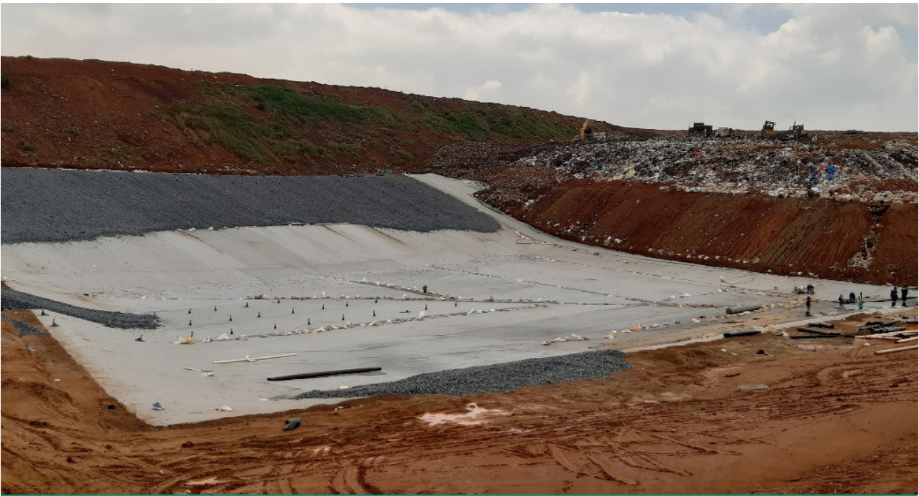
The Waste Group Class B liner being completed at the Mooiplaats landfill site in Centurion, Gauteng
