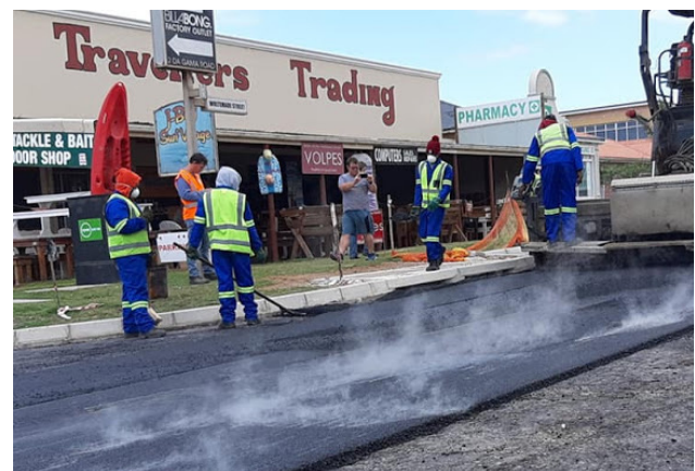
A street in Jeffreys Bay is repaired by making use of plastic waste.
