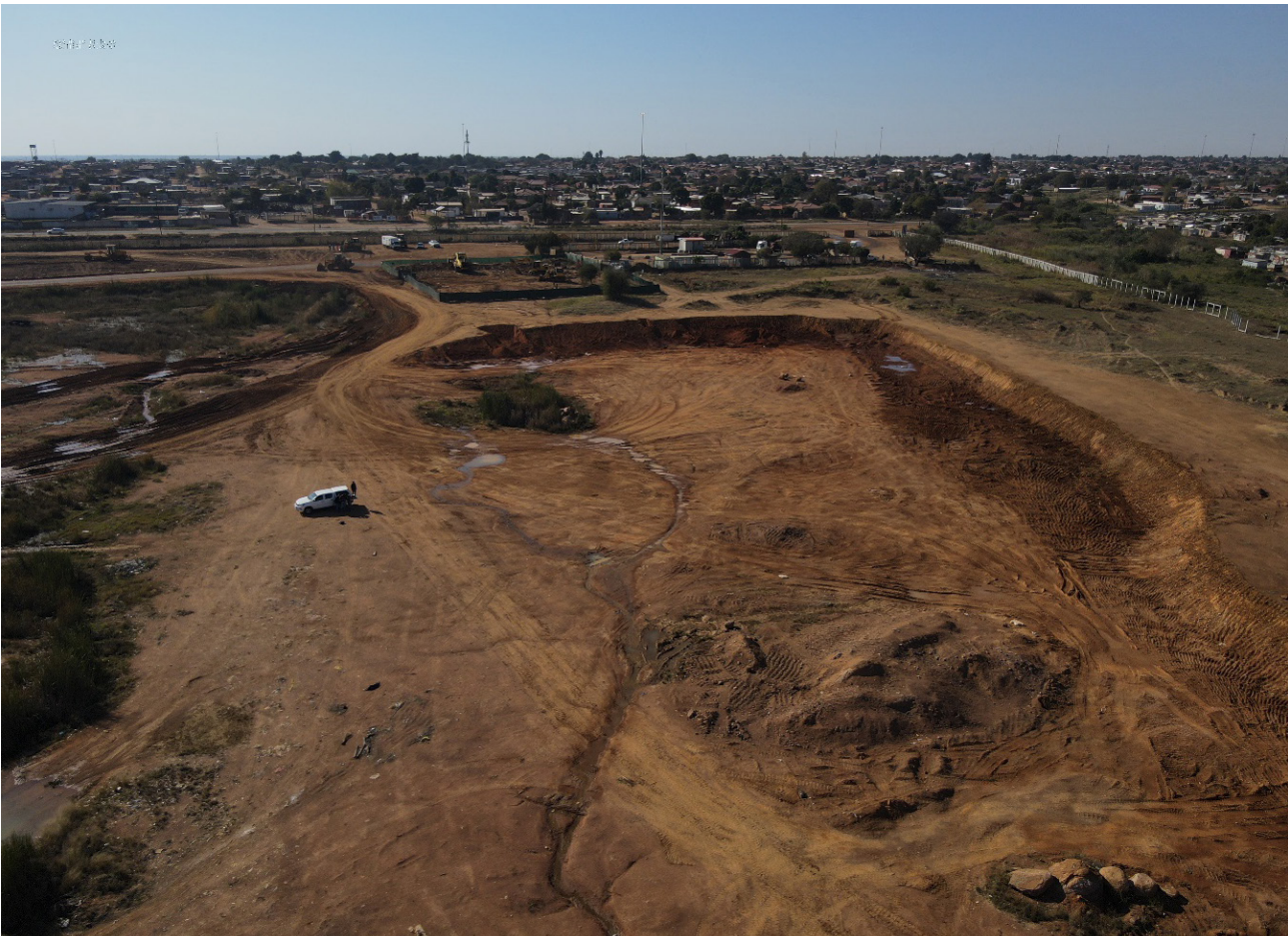
Aerial view of a wet weather cell
