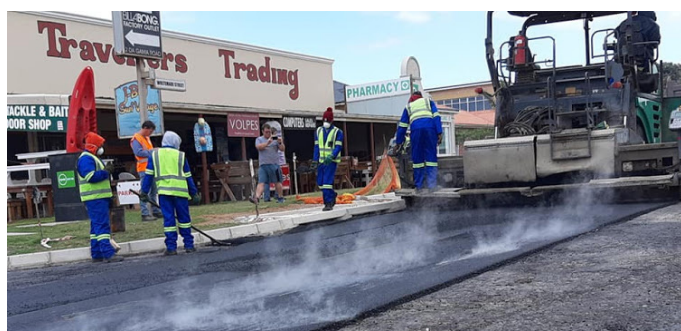
A street in Jeffreys Bay is repaired by making use of plastic waste.
