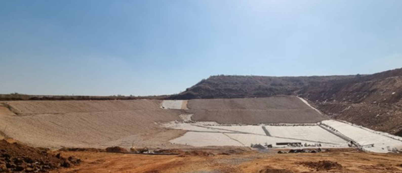
The Waste Group Class B liner being completed at the Mooiplaats landfill site in Centurion, Gauteng.
